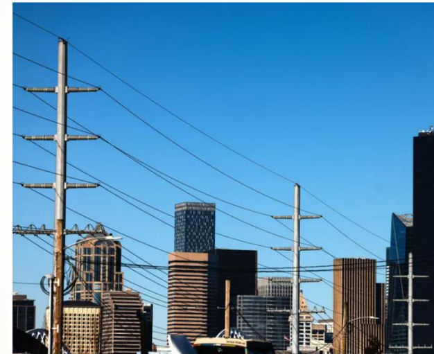
Power lines seen in the Sodo area in Seattle in January 2025. (Karen Ducey / The Seattle Times)
